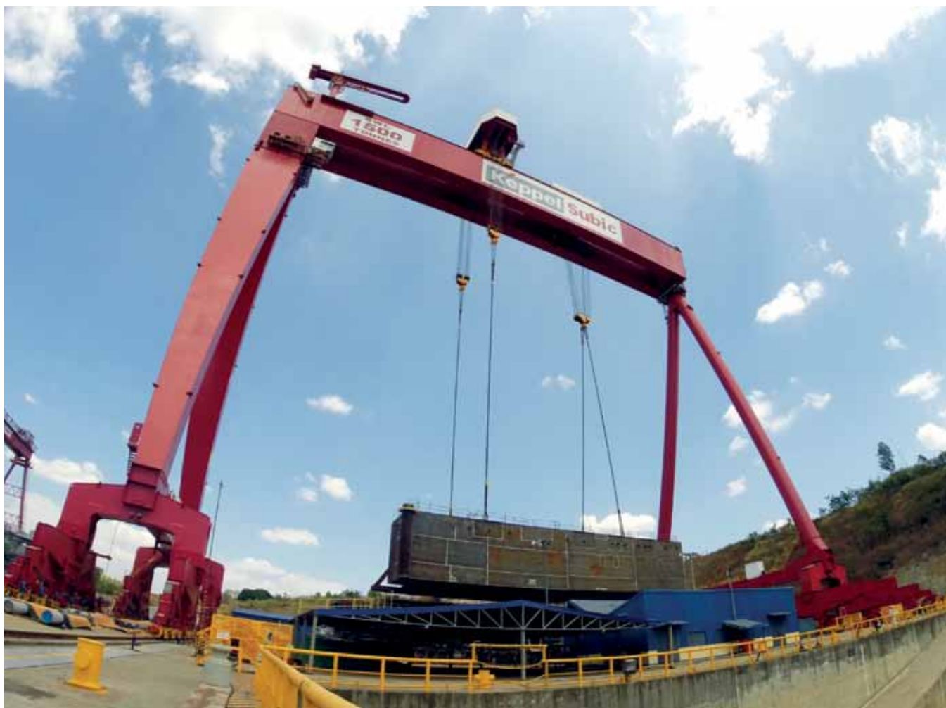
The 1,500-tonne gantry crane at Keppel Subic Shipyard has been supporting the installation works of the DCP that the shipyard is building for Shell Philippines Exploration
