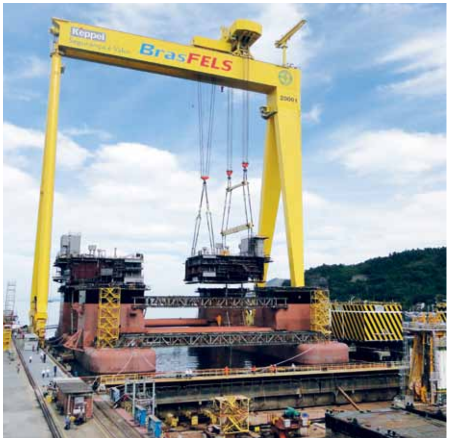
BrasFELS' newly installed 2,000-tonne gantry crane is supporting the installation of megablocks for a DSS™ 38E semisubmersible project
