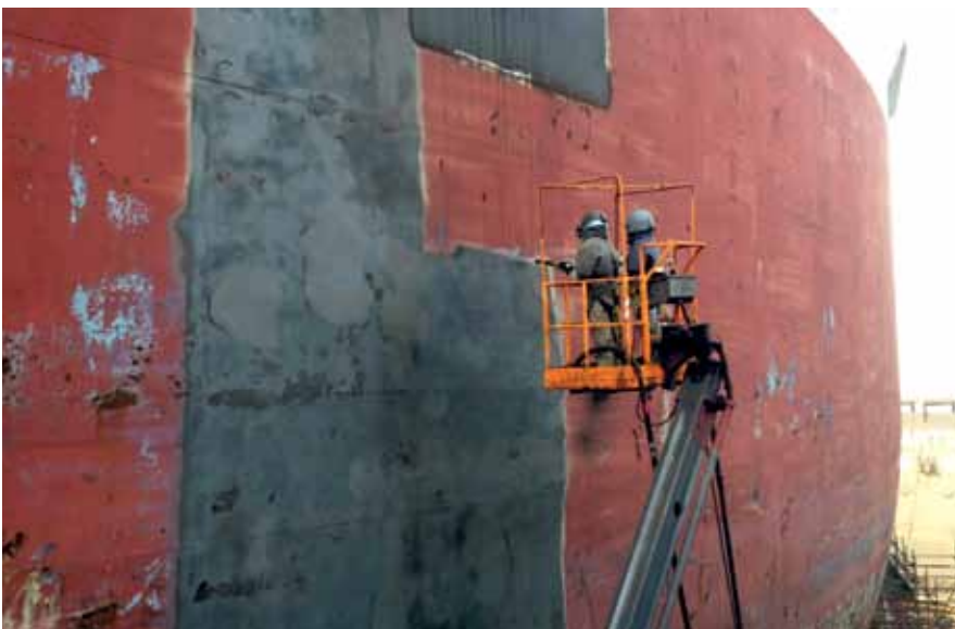
The new semi-automated blasting system allows workers firing the blasters to control output of the blasting material directly instead of relying on other workers to do that. This results in savings in grit usage as well as higher productivity
